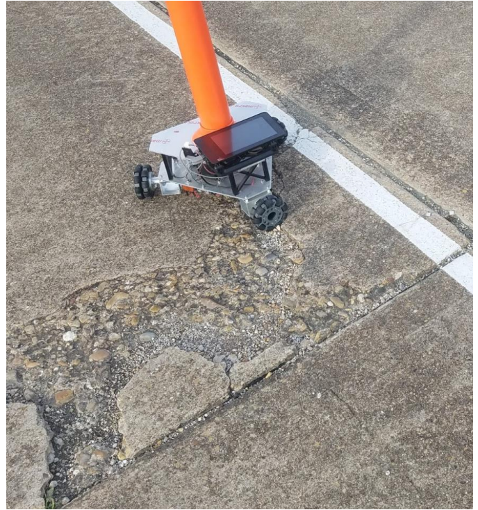
Figure 7. Surface Defects seen by Platform
