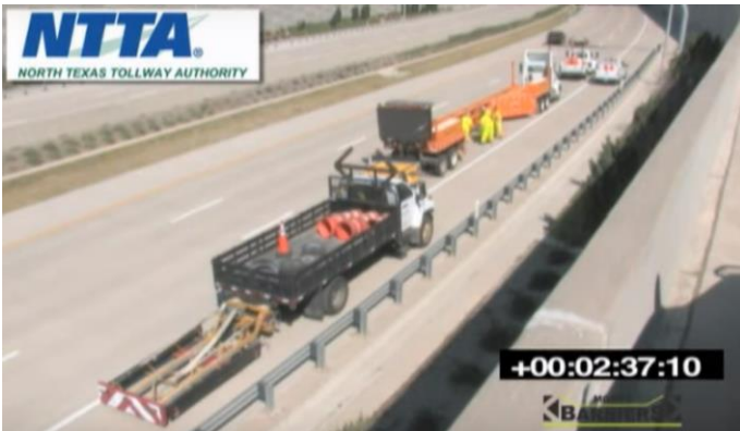
Figure 1. Attenuator Truck (orange) with Service Truck (black)
